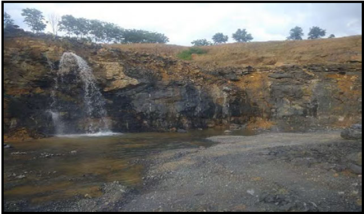
Fig.4: Accumulation of seepage Water in front of the Blasting Benches
